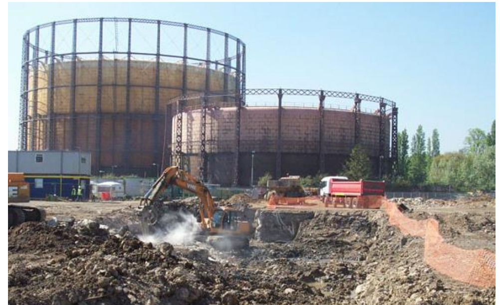
Contractor photograph from the 2002 remediation of the western half of the site
